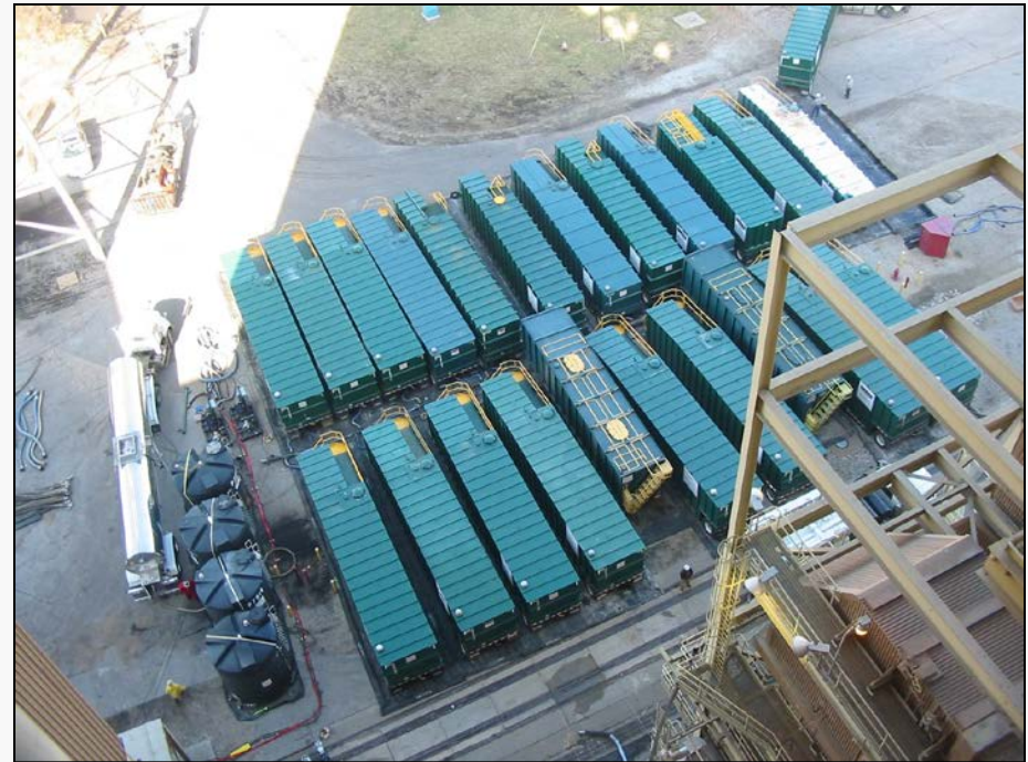
Boiler chemical cleaning tank farm
