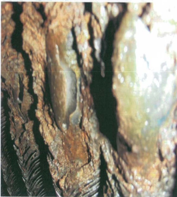
Frozen Tube Damage
