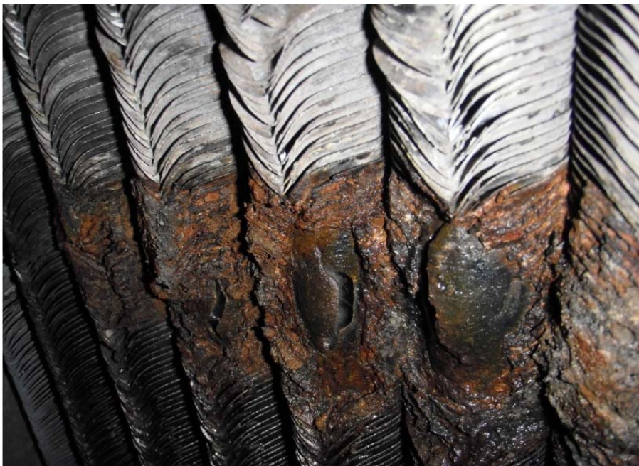
Corrosion Build-up Behind Support Beam
