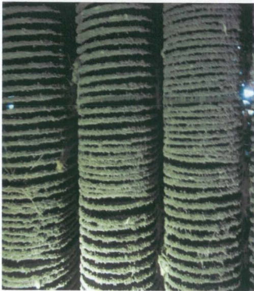
Severe Debris Build Up on Tube Fins
