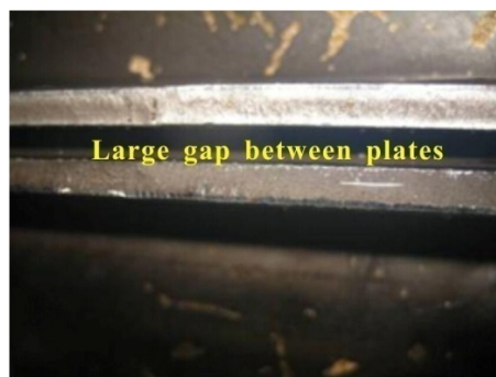
Figure 1. Gap between water distribution plates (Influent)
