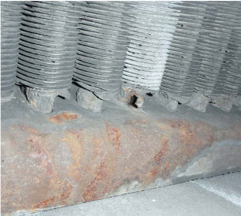
Holes in Tube Headers
