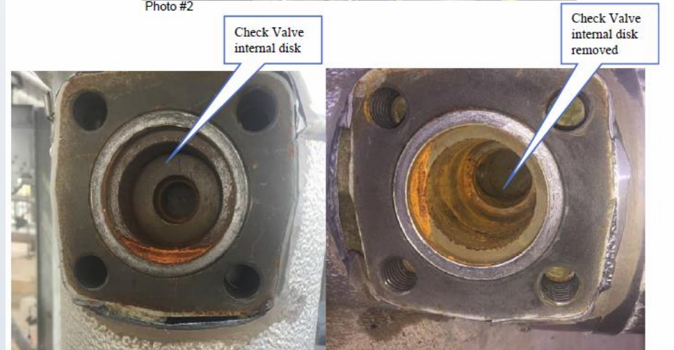
Photo #3) Check Valve Internal disk rusted in place.
