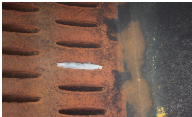
Upper steam distribution duct 5 Feedwater treatment regime: AVT(O) DHACI rating = 1
