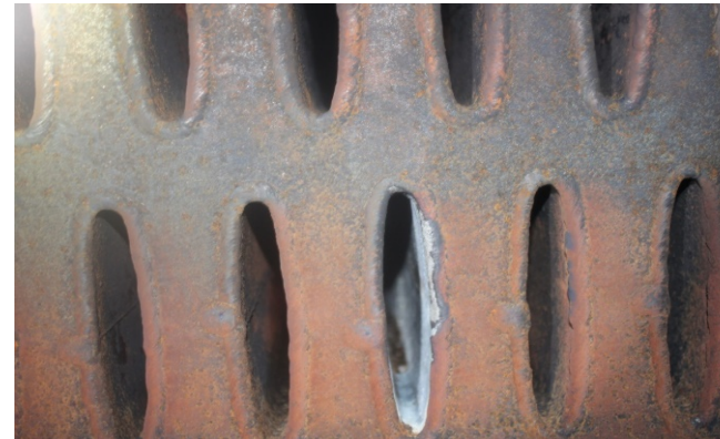
Upper steam distribution duct 5 Feedwater treatment regime: AVT(O) DHACI rating = 4
