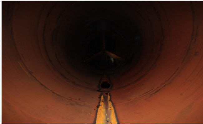
LPT 1 exhaust duct Feedwater treatment regime: AVT(O) DHACI rating = A
