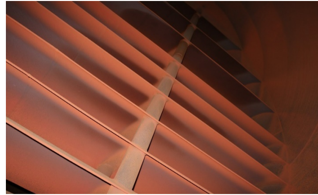
Steam distribution duct 1 inlet louver Feedwater treatment regime: AOT DHACI rating = 1
