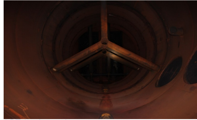
LPT 2 exhaust duct Feedwater treatment regime: AVT(O) DHACI rating = A
