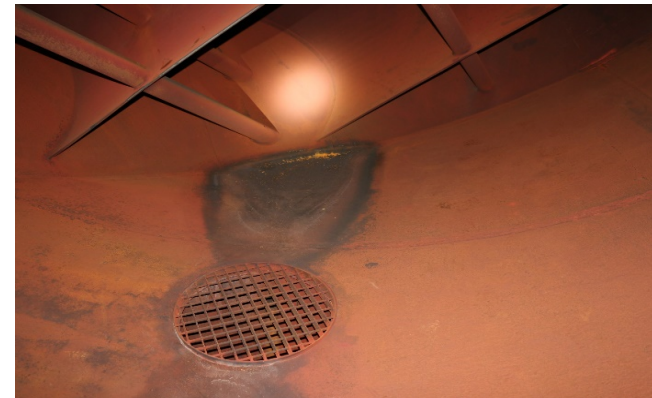
LPT 1 exhaust duct Feedwater treatment regime: AOT DHACI rating = A
