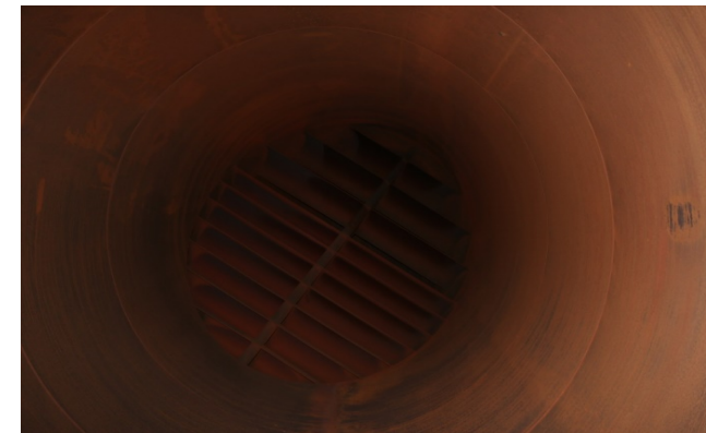
Steam distribution duct 3 Feedwater treatment regime: AOT DHACI rating = 1
