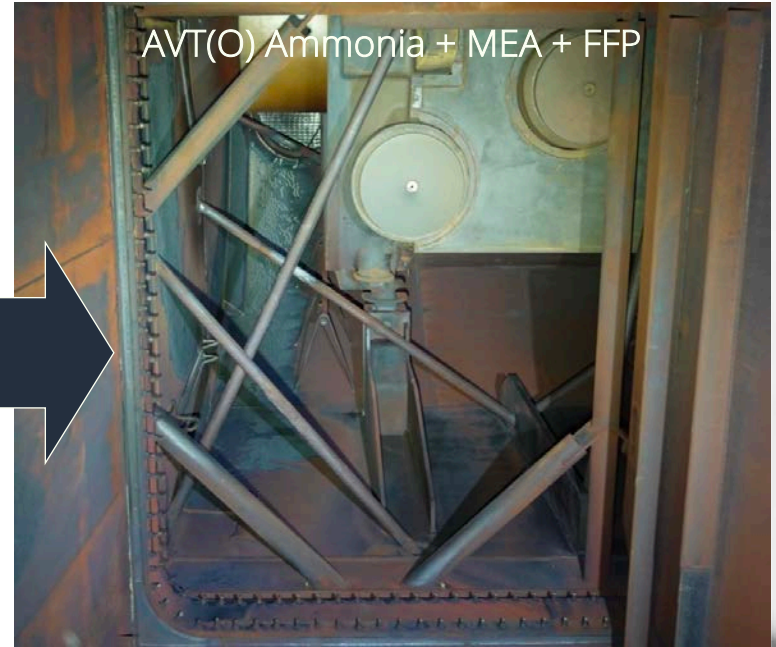
FAC ductwork LP turbine Tiger striping
