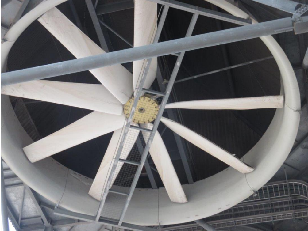
Figure 8: Broken and missing fan blade
