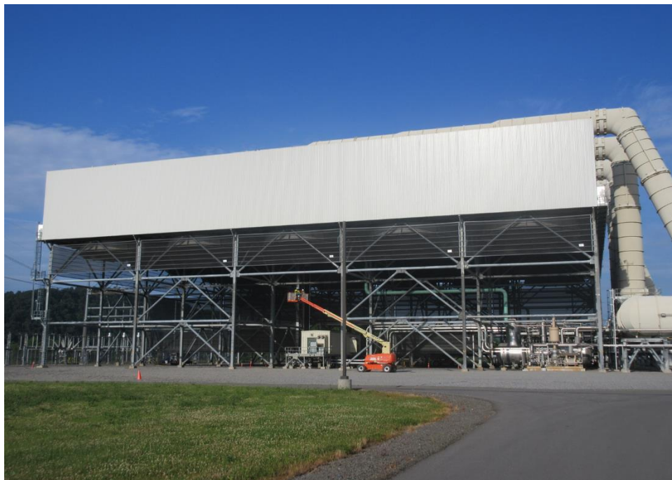
Figure 15: Combination of perimeter screen to reduce stress on fan blades and cruciform screens to reduce wind induced performance deficiencies
