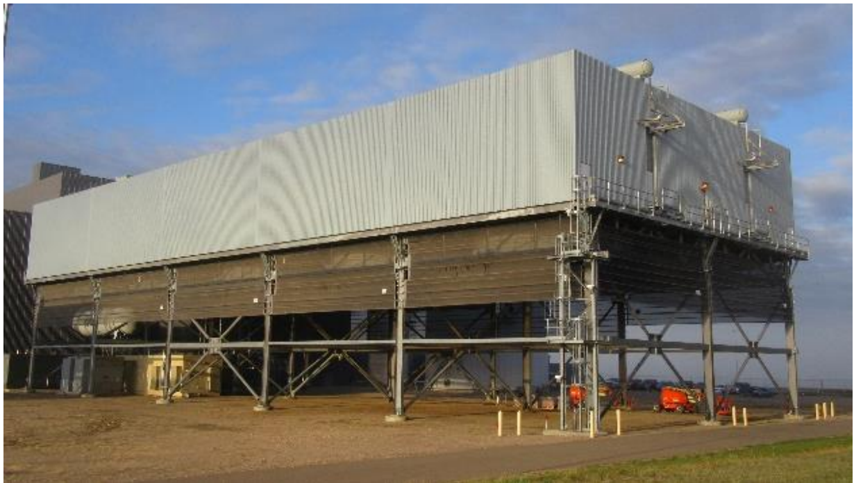
Figure 11: Perimeter screens to reduce vibrations and fan blade damage
