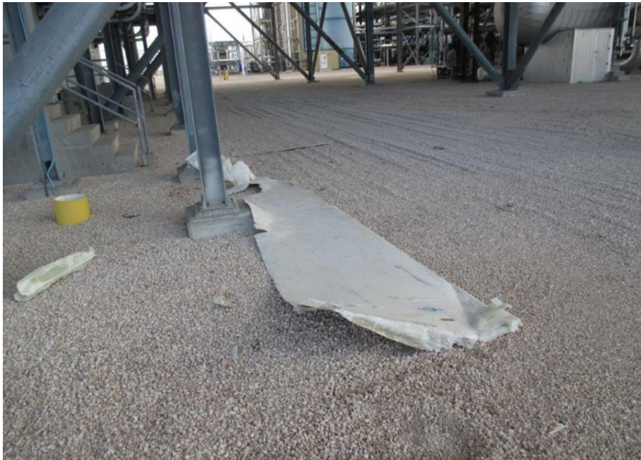
Figure 9: Failed fan blade on the ground; this represents a significant potential safety hazard for personnel working underneath the ACC.
