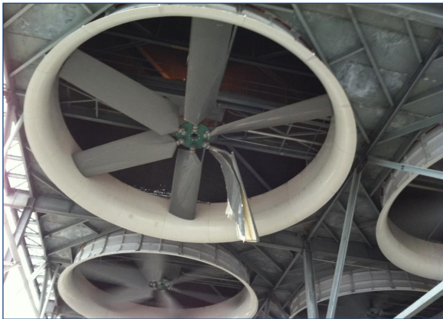
Figure 7: Broken fan blade due to dynamic blade stress
