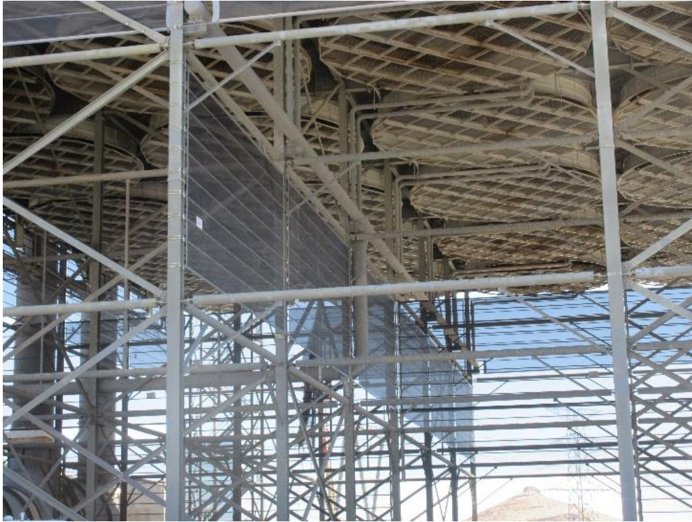
Figure 12: Internal screening to prevent crosswind losses to fan airflow
