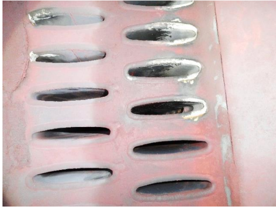
Figure 16: Significant corrosion ('bare metal') at thin-walled finned tube entries
