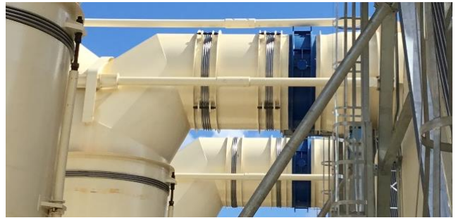
Figure 13: Flanges / expansion joints ACC risers
