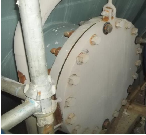
Figure 15: Manway entry cover, inadequate bolt torquing
