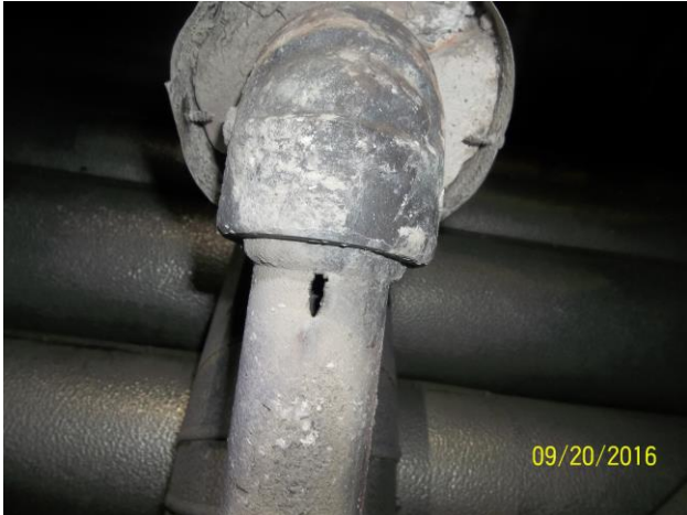
Figure 20: Leak resulting from corrosion under insulation
