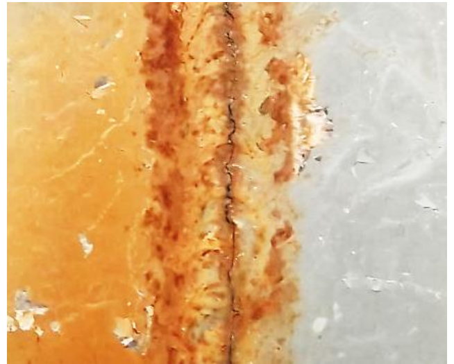
Figure 9: Crack in repair of ACC duct
