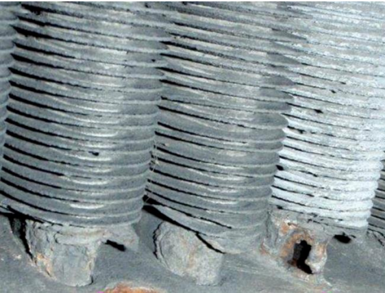
Figure 17: Through-wall exterior corrosion at lower tube due to cleaning water quality
