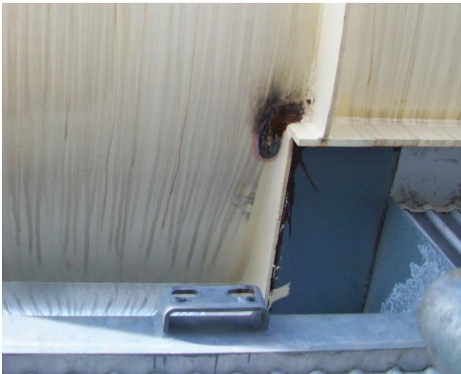
Figure 11: Local rust may indicate wall penetration.
