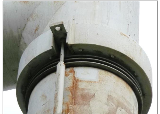
Figure 14: Leak at expansion bellows in riser duct
