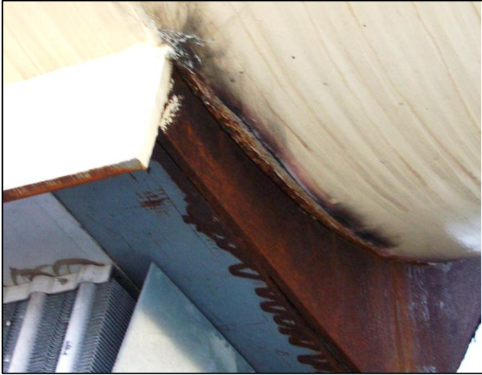
Figure 10: Attachment weld to steam distribution duct
