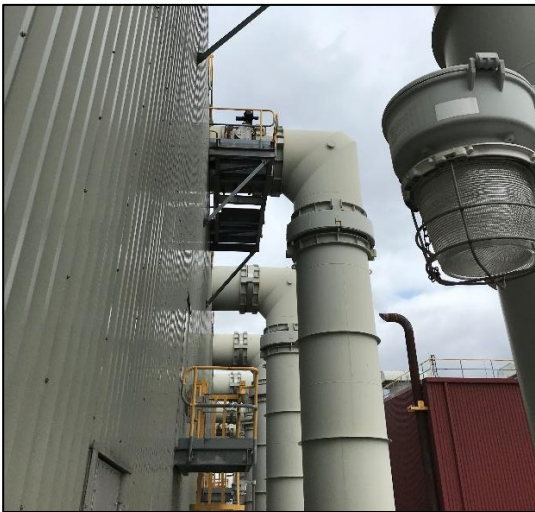
Figure 7: Access to exterior of risers for leak testing is challenging
