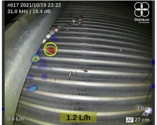
Figure 4: Acoustic detection of a leak in ACC tube
