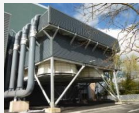
Combined Cycle Power Plant in UK
