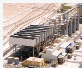
Combined Cycle Power Plant in Middle East
