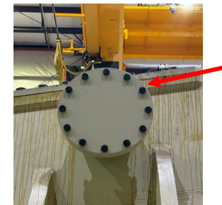
LP Hood Manway
