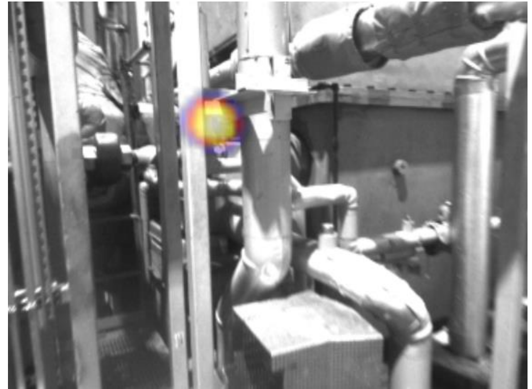
Turbine Shaft Seals
